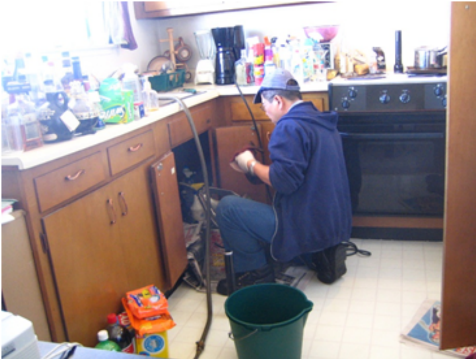
“Plumber at work” by photo taken by flickr user rick - Flickr. Licensed under CC BY 2.0 via Commons -
